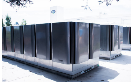
4 fuel cell installations 13.75 MW
