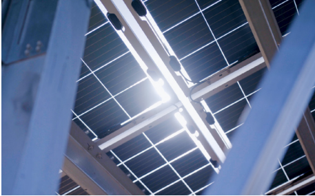
10 solar installations 8.7 MW
