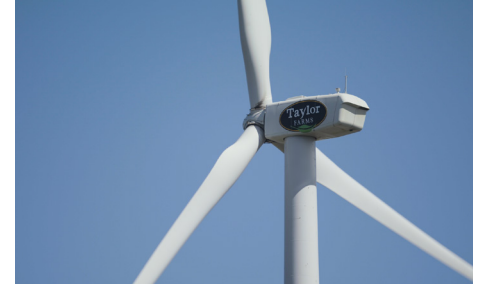
1 wind turbine 1 MW
