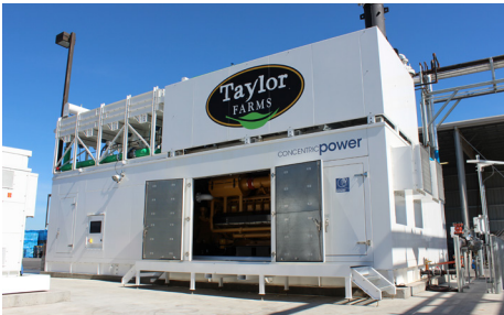
1 cogeneration system 2 MW
